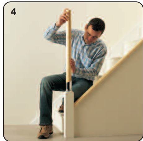
4 After measuring your post to the correct length, fit and secure the posts in place. Repeat for all newel posts.
